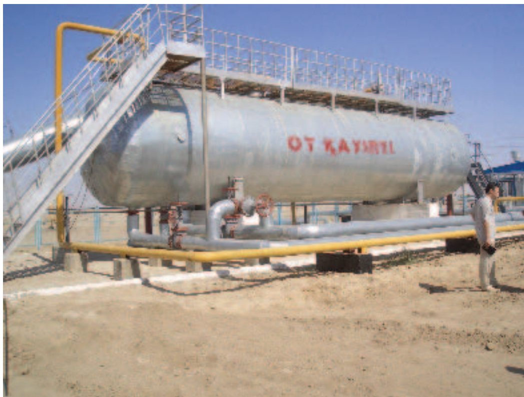
Uzen Field NGDU 3 Group Unit 65 Three Phase Separator
