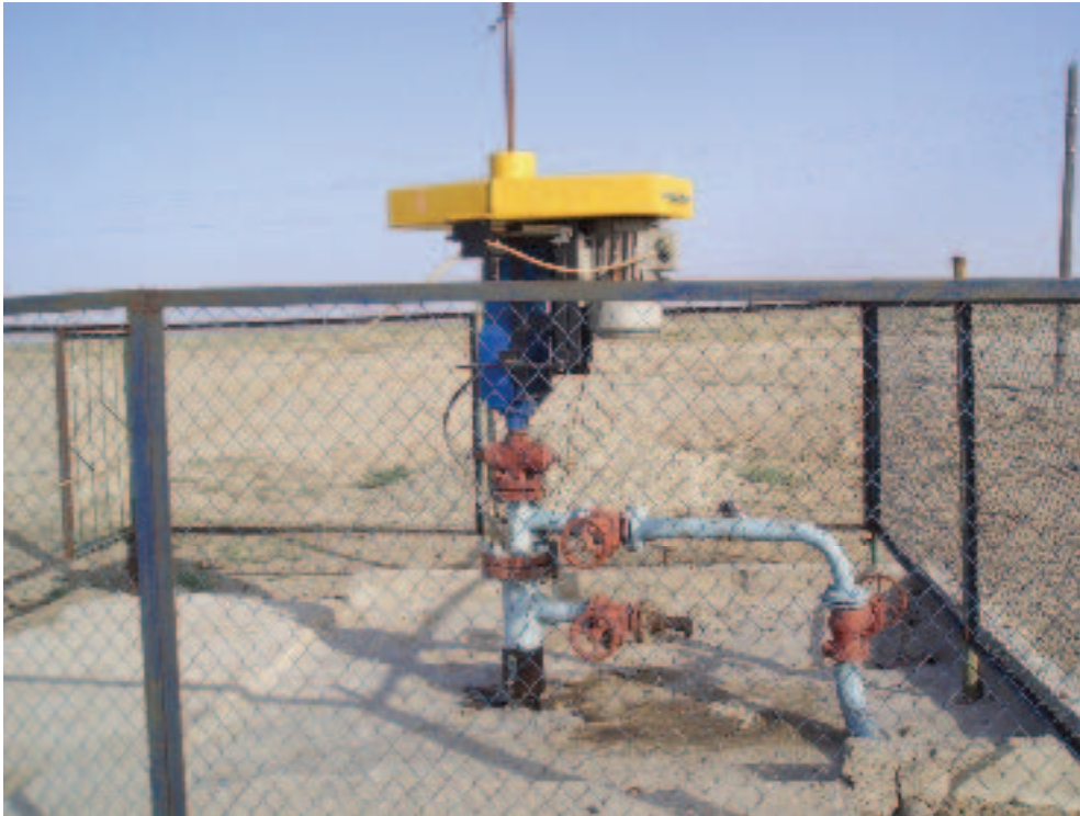
ZhaikMunaiGas NGDU Gran Field Screw Pump Oil Well
